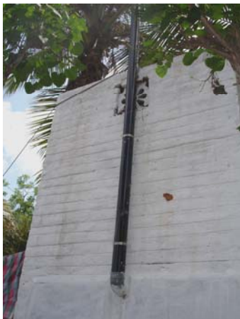
Black painted Vent Pipe .
